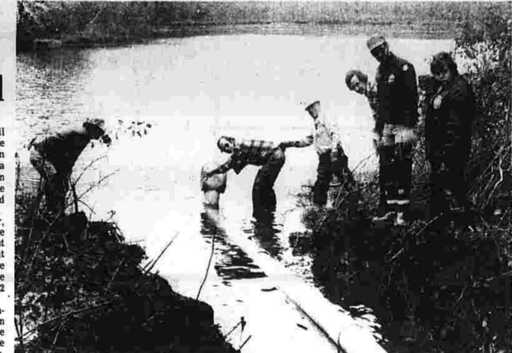
Volunteer Work Several members of the Bolton Volunteer Fire Department worked last Saturday to install a dry hydrant in the pond off Bayberry Road. The department members will install a second dry hydrant in Dimock's Pond, off
